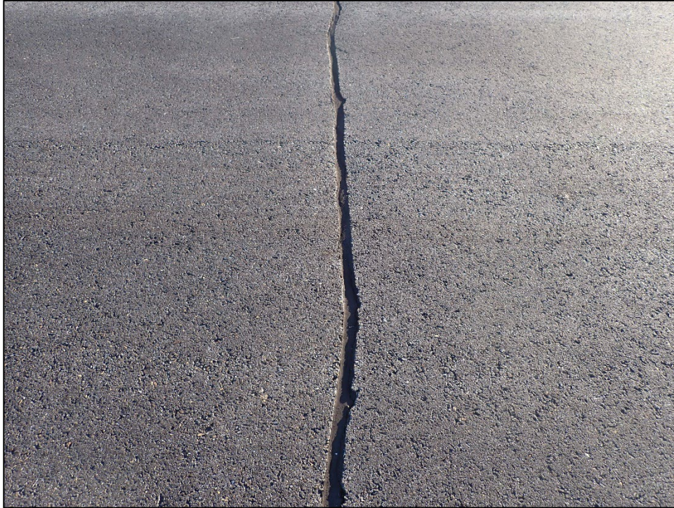
RW14-11-49: L&T Cracking
