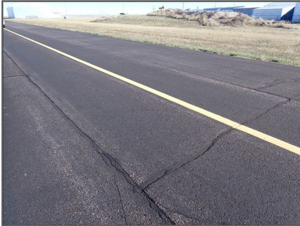
TW-05-10: L&T Cracking
