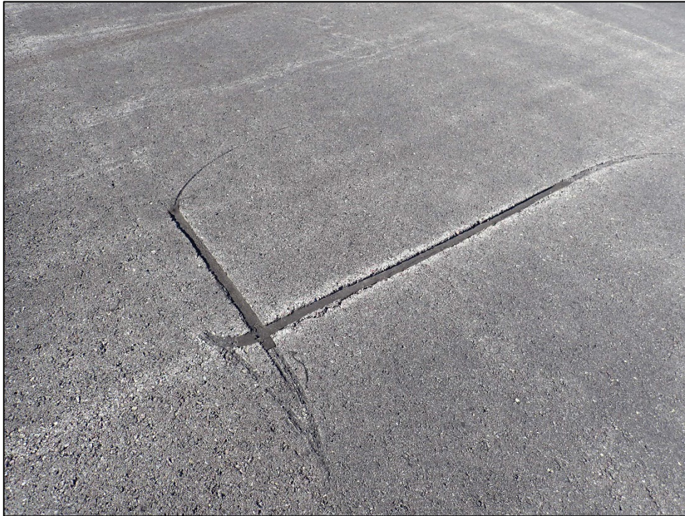
AP-01-18: L&T Cracking
