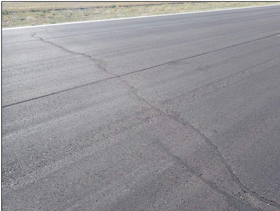
RW05-21-41: L&T Cracking
